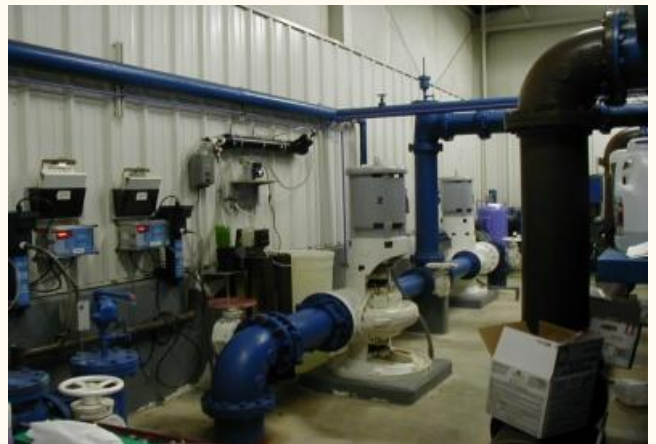
The Water Treatment Plant's Turbidity Meters
